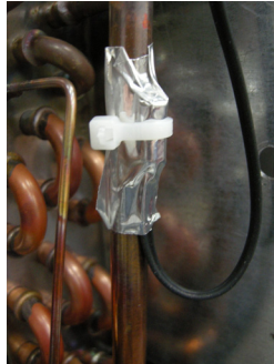
Thermistor attached to the refrigerant line.
